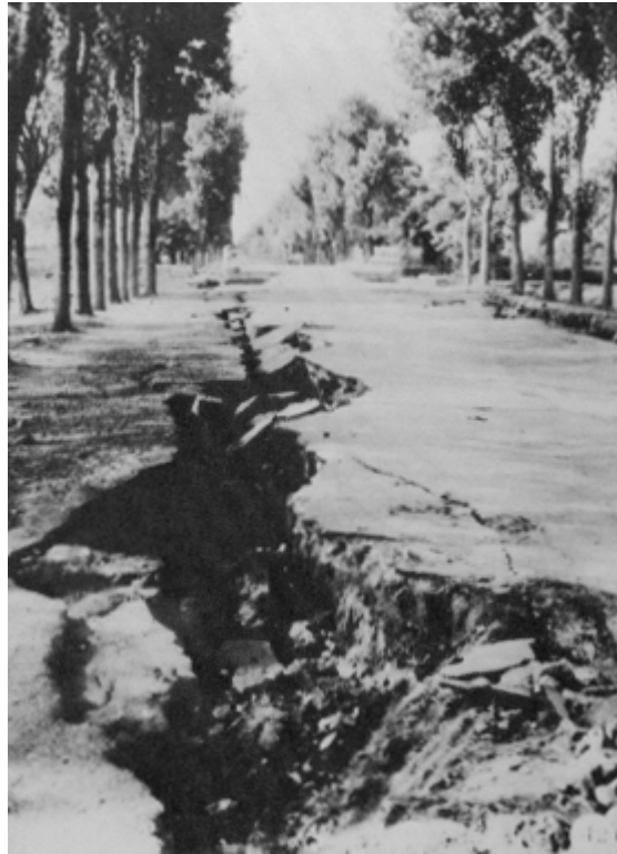
Figure 81. Damage to a road caused by soil failure.
