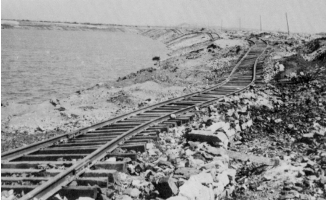
Figure 22. Failure of ground under railway line. Extensive damage was done to the rail system in the Tangshan region.
