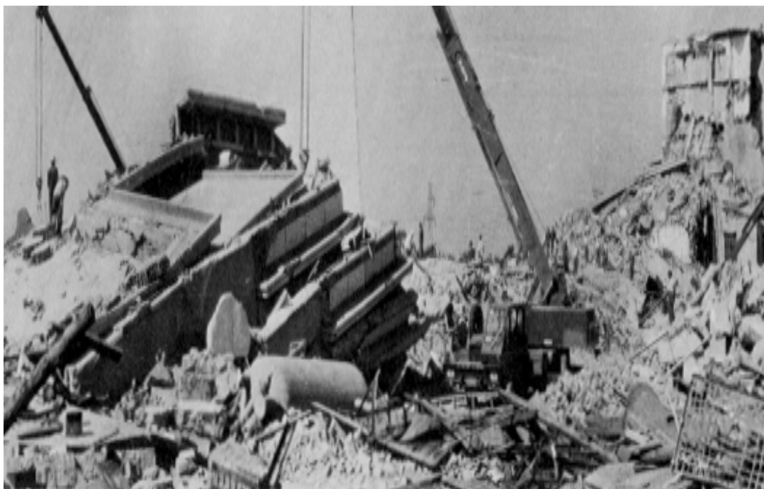
Figure 42. Collapsed out-patient service building of the Kailuan coal mine general hospital, Tangshan.
