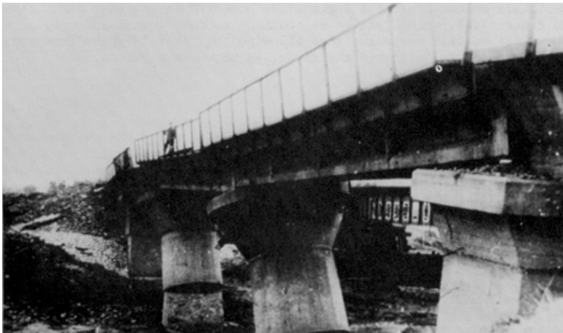
Figure 75. Tilted piers and broken abutment of the railway bridge on Tangshan-Kenhua Line.
