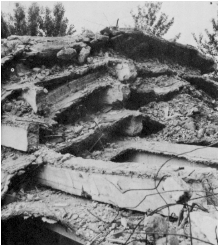
Figure 45. Collapsed five-story physics-chemistry building of the Tangshan Mine-Metal Institute.
