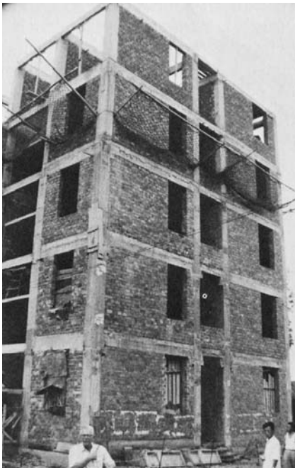
Figure 13. End wall of the five-story wing of the Chengdu office and storage building. The brick walls are lightly reinforced shear walls.
