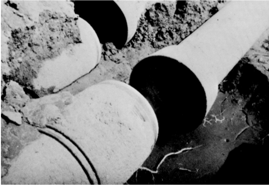
Figure 24. Underground pipes separated by extensional ground deformation.
