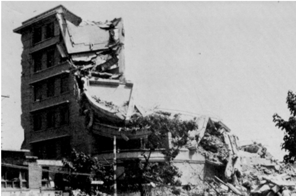
Figure 48. Collapse of six-story building at the Kailuan coal mine hospital, Tangshan.
