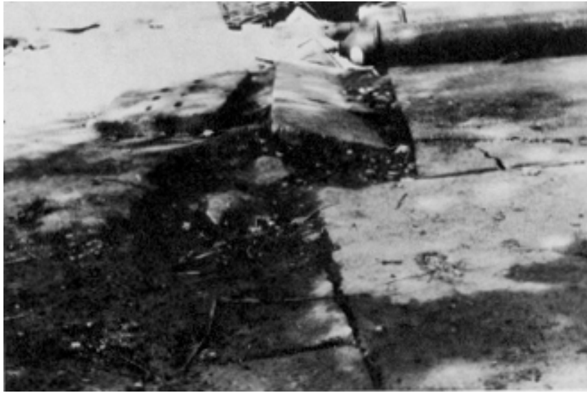
Figure 36. Surface breaks and compressed pavement over drainage trench in Tangshan
