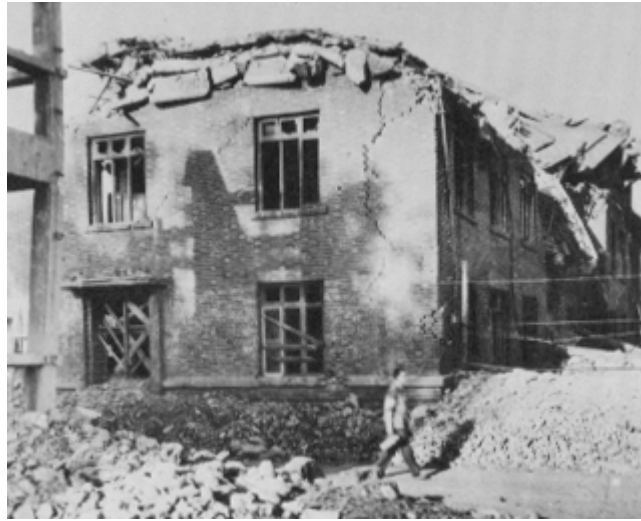
Figure 64. Partly collapsed five-story building at Coal Mine Design Institute in Tangshan.
