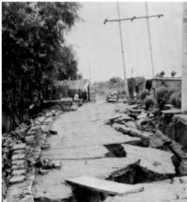
Figure 23. Damage to road near Loting Hsien. Slumping, lurching and settlement of soft soils caused extensive damage to highways in the Tangshan region.
