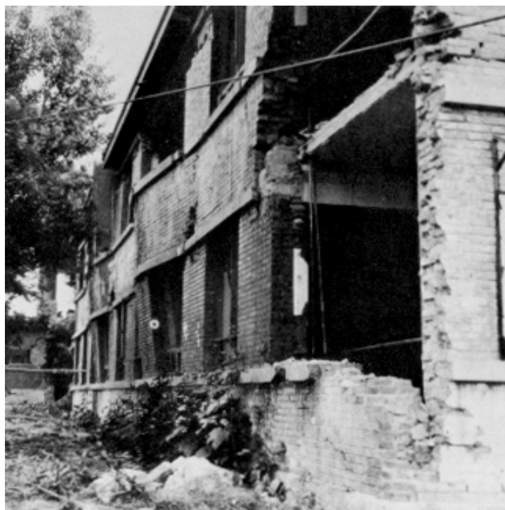
Figure 54. Badly distorted brick building on the verge of collapse. The second floor appears to be of precast concrete slabs supported on precast concrete beams, which, in turn, are supported on unreinforced brick piers.
