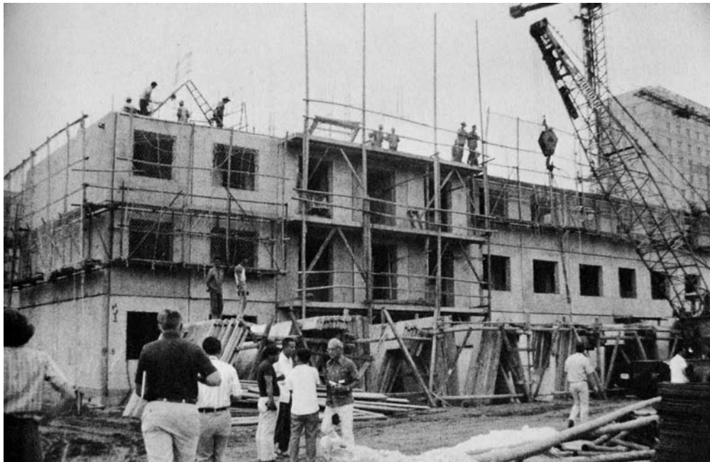
Figure 2. Exterior view of apartment building in Beijing in an early stage of construction in the summer of 1978. The exterior walls are precast, while interior walls are cast-in-place.
