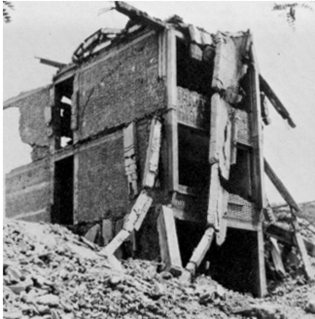
Figure 47. Collapsed five-story office building, Tangshan. The lower three stories had concrete columns, and the upper two stories were unreinforced brick without concrete columns.
