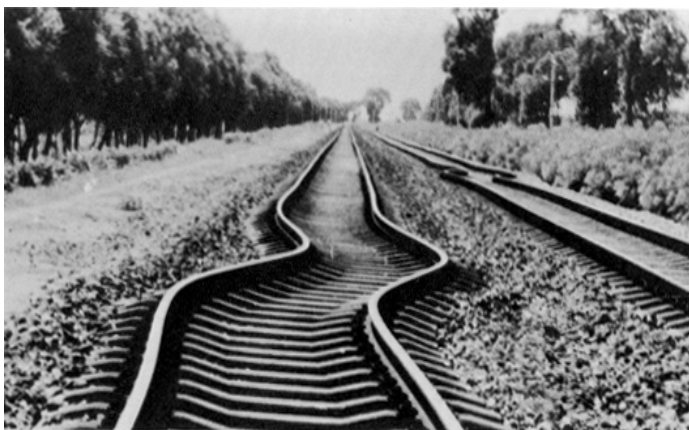
Figure 21. Buckling of rail lines due to ground deformations. The general Tangshan region had many soft soils that behaved poorly during the earthquake.
