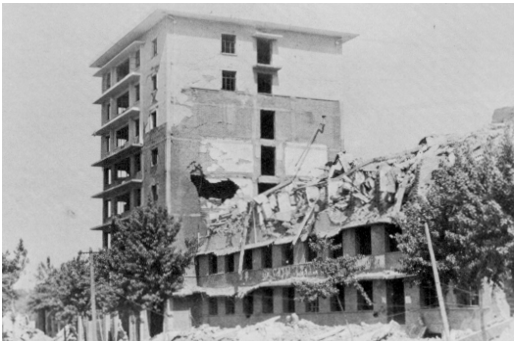
Figure 50. Eight-story Hsinhua Hotel in Tangshan was badly damaged at the fifth-story level but remained standing. In the foreground is a collapsed six-story building.
