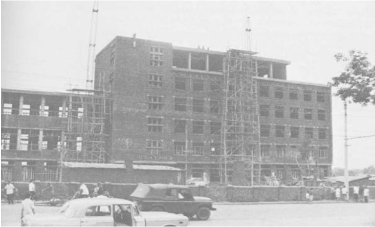
Figure 5. Exterior view of six-story brick walled building in Harbin. The structure was intended to house an electronics factory when completed.
