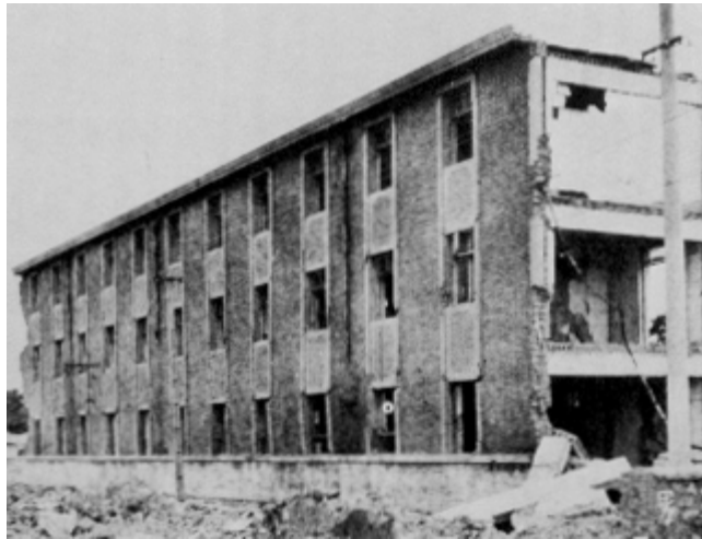
Figure 69. Damaged car factory dormitory building in Tangshan. The first story was most severely damaged but the building remained standing.
