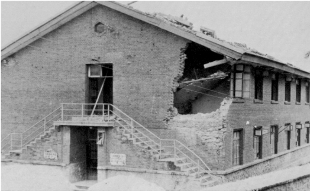
Figure 68. Damaged Tangshan second reception building. Although damaged, this two-story brick building remained standing.
