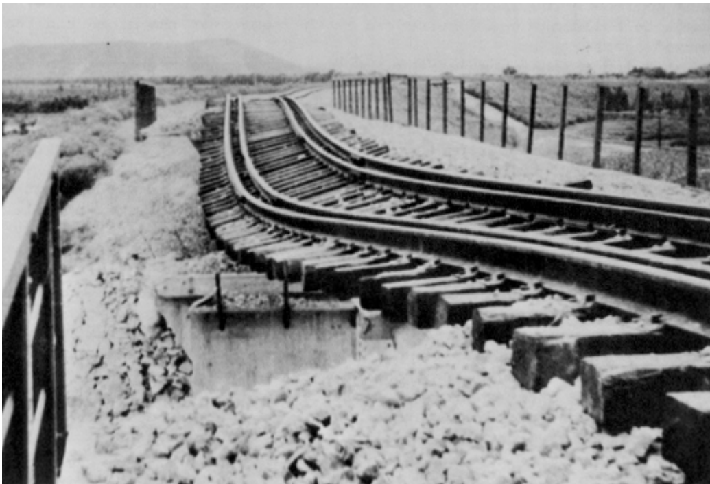
Figure 82. Damage to railway line caused by loss of support.
