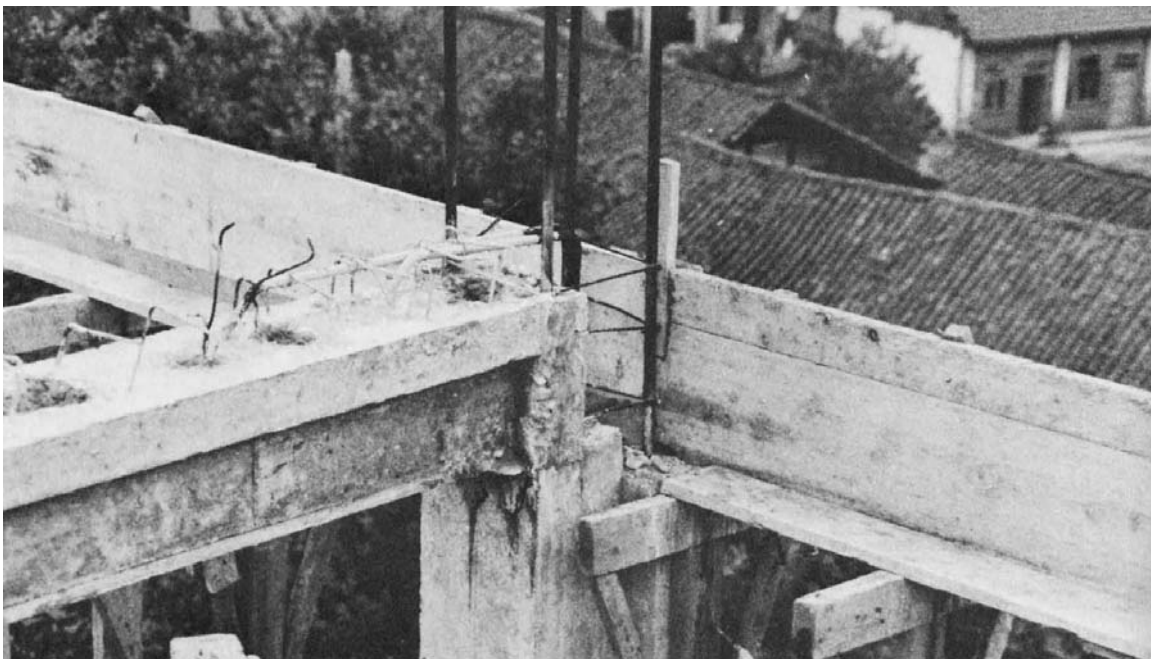
Figure 16. The columns and transverse beams have been cast in place in this detail of an upper floor. Forms are in place for the cast-in-place spandrel beam. The joint is integral but a construction joint goes through the center.
