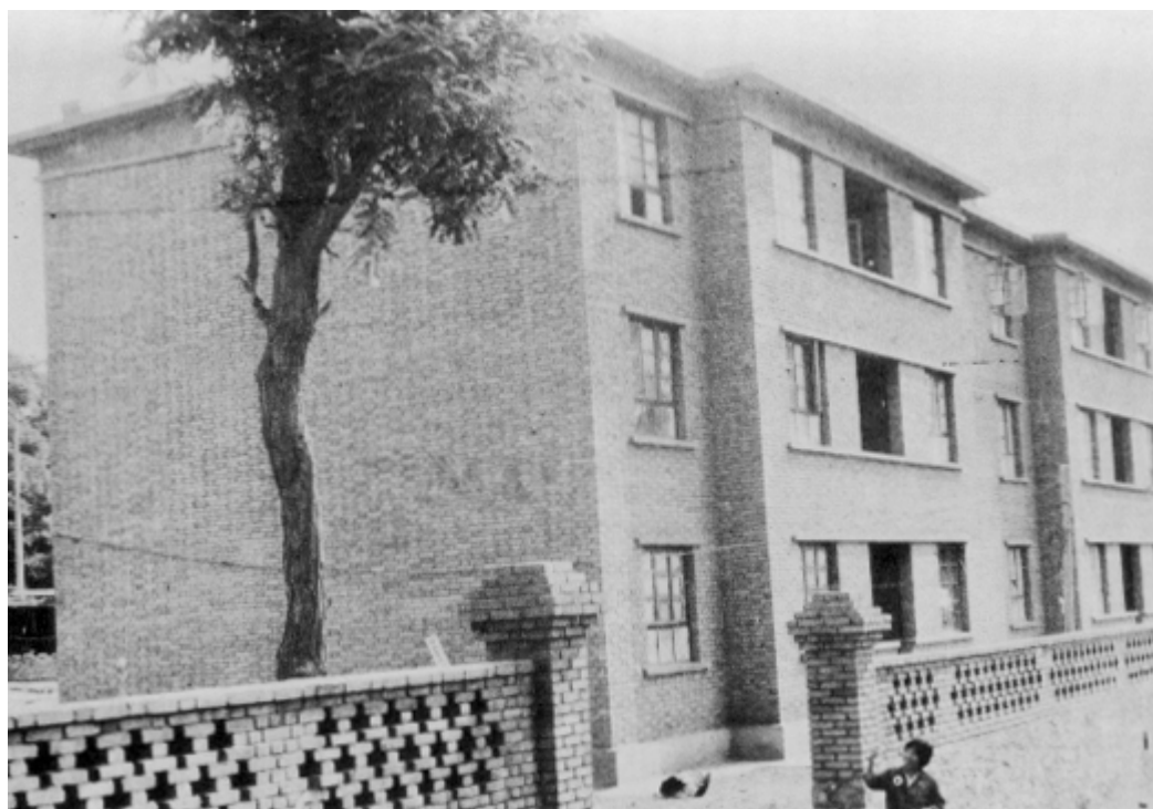
Figure 71. Cement factory worker apartment building 422. This structure was located on bedrock north of Tangshan and received only slight damage.
