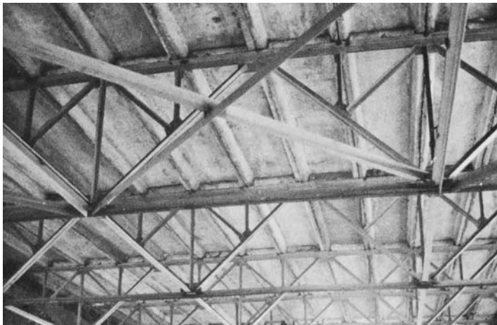
Figure 6. Harbin electronics factory. The roof over the small auditorium has steel trusses supporting precast concrete channel sections.
