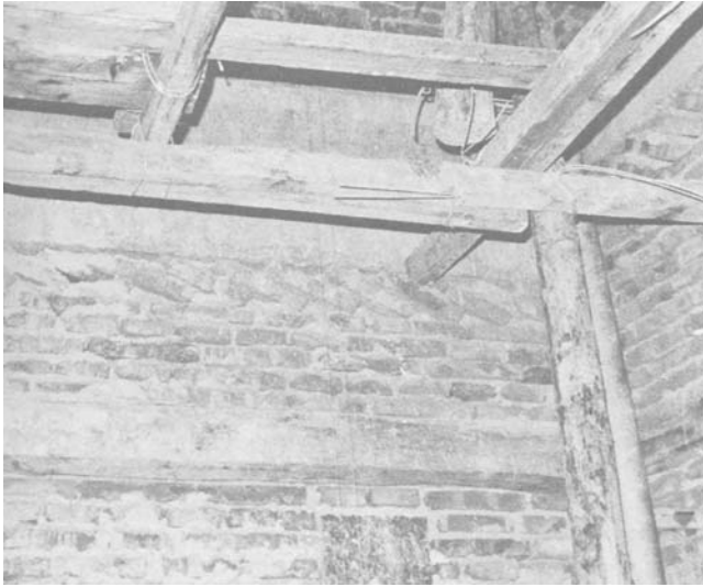
Figure 4. Interior of elevator shaft of Beijing Duck Restaurant showing brick filler walls. Note “leaning soldier” bricks at top, a method of filling space that is not a module of brick dimensions.
