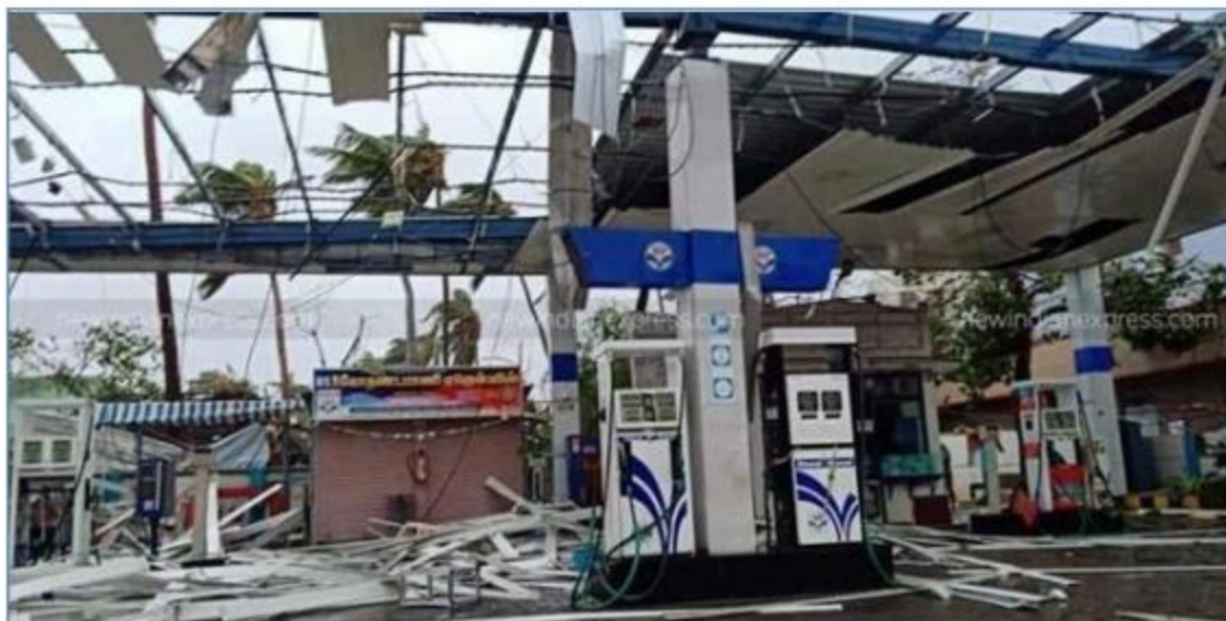
A destroyed petrol station in Velankanni, Nagapattinam district (Source: newindianexpress.com)
